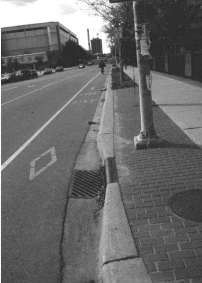
Narrow gutter, wide drain in Madison, WI.
