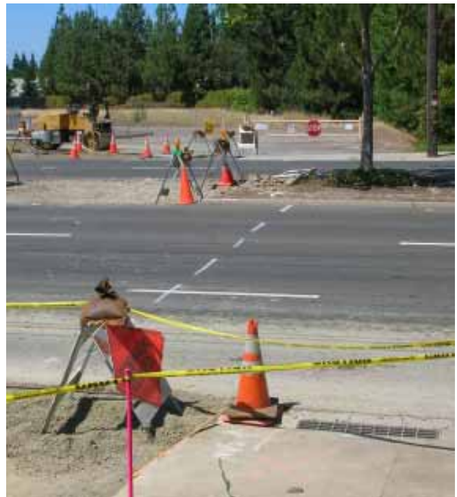
Construction is under way for a bicycle/pedestrian signal where the Folsom South Canal trail crosses Sunrise Boulevard. Photo by Lea Brooks
